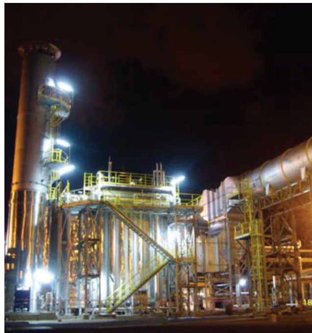
Petronas Gas, Compressor Station
