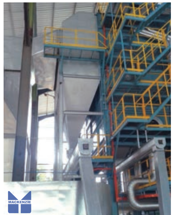
Dust Collector System
